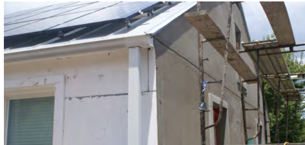
Figure 2. Completion of the insulation system (EIFS) and installation of the PV system on the unit roof
